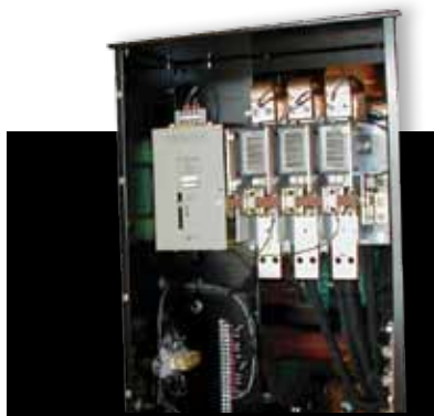
Generator Paralleling Switch
